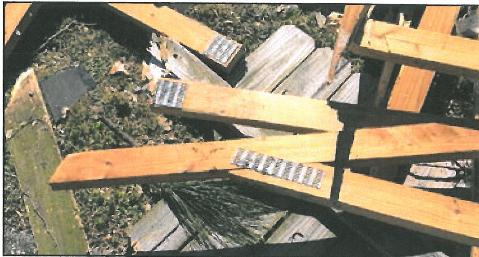
No clips on any of the trusses from the debris pile of this home (non-REBUILD home).
