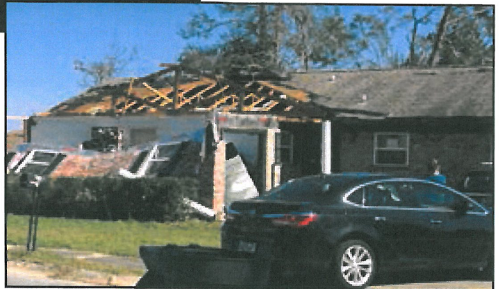
Garage door failure likely led to rapid pressurization of home (non-REBUILD home).
