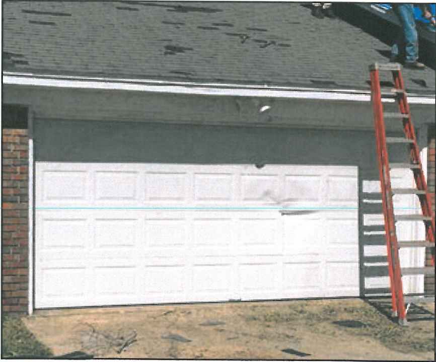
REBUILD home with a new garage door impacted by a tree.
