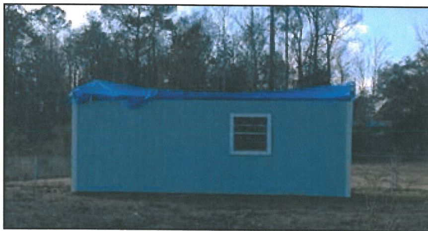
Roof-to-wall failure of an out-building (not hardened by REBUILD) on the property of 111 Upton in Century
