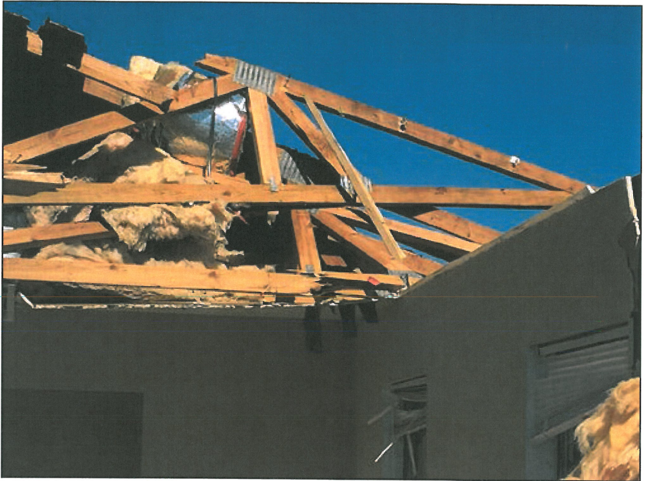
No clips on any of the trusses on this non-REBUILD home
