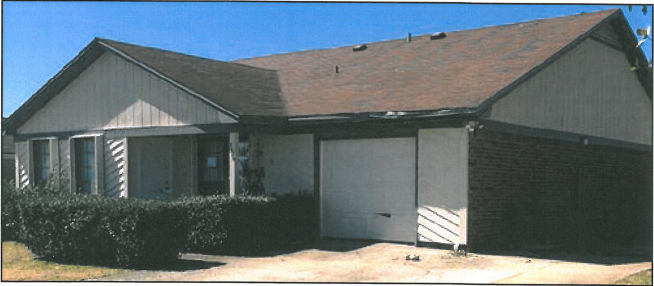
REBUILD home with a new garage door impacted by windborne debris from the destroyed home across the street.
