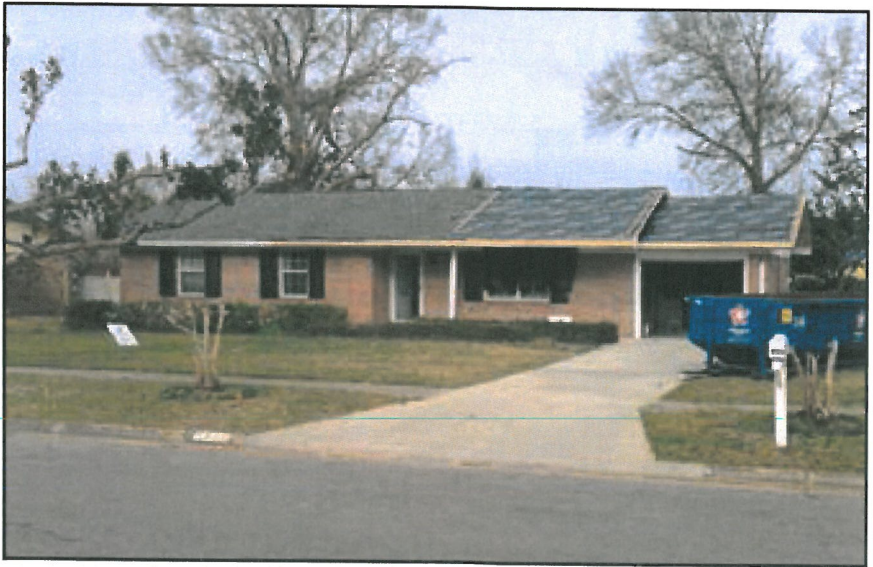
Front view of 7800 Le Jeune Drive. This home had been repaired and was being re-roofed at the time of our inspection. Note that the gable-end-bracing REBUILD had installed on the garage gable held, preventing the gable truss from failing and causing more extensive damage.
