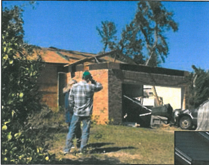
Garage door failure likely led to rapid pressurization of the garage on this non-REBUILD home.
